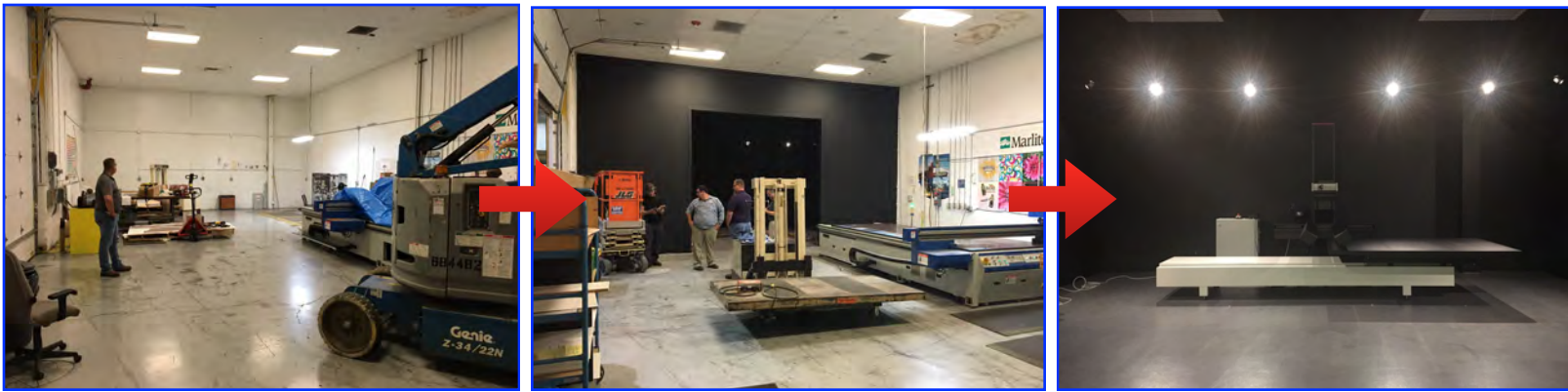
Progress is being made at a rapid rate on the new Digital Print project. The scanner is in and functioning. Demolition of the area for the print line is complete.
